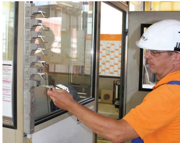
Wolfgang Schüle (Head of Maintenance) demonstrates the removal of the keys at the control room.
