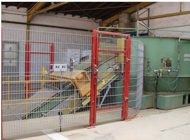
Safety fences protect from the dangerous plant components in material processing.
